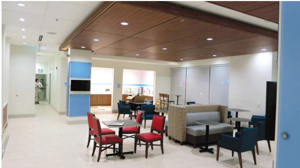
Here is Sargent’s team putting the finishing touches to the foyer at the Holiday Inn Express
